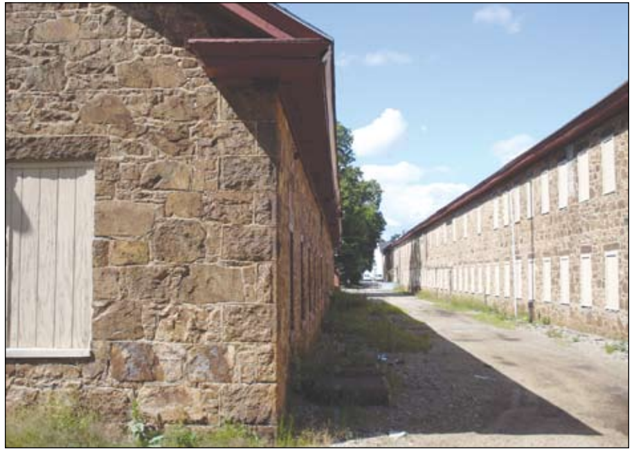
The 1868 Antrim Opening Shop on the left is one of nine granite buildings built between 1852 and 1907. It is threatened with total demolition as part of the new development. Photo courtesy of Chris Milford.
